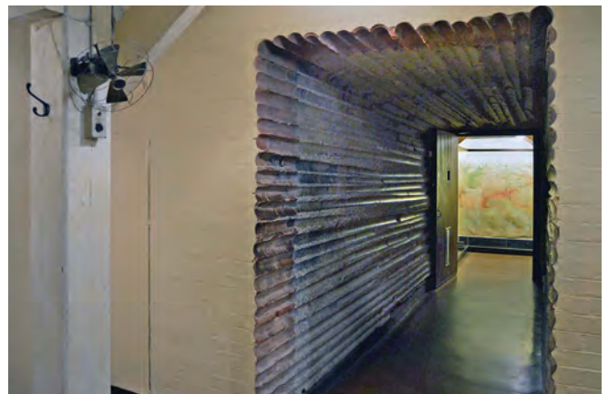
Cored hole through concrete-filled room under stairwell to allow postwar access around the complex. The wartime concrete was unreinforced but sufficiently hard to take the workmen many times longer to drill than they had planned
